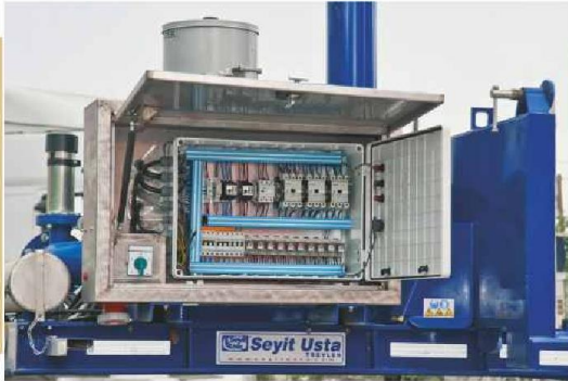
Electric control panel stored in stainless steel box to avoid impacts
